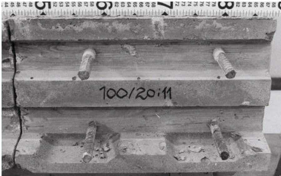
Figure 6 Beam end with 20 mm cover to the rebars at the bottom.
